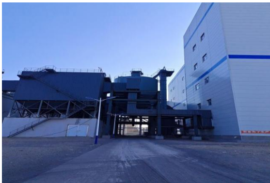
渣仓布袋除尘器+26.5m 排气筒 (DA006)
